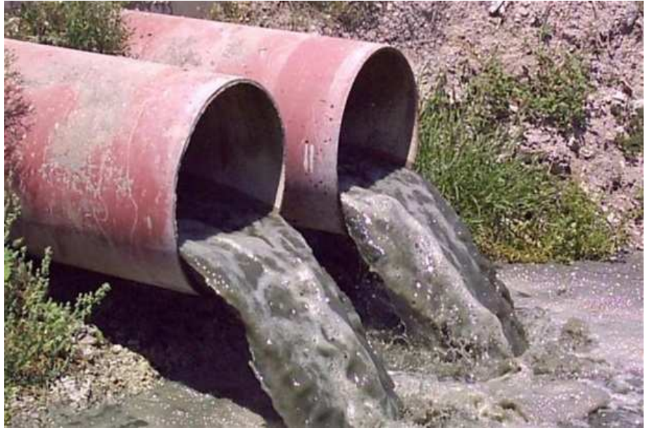
Pic 6. Water contamination
