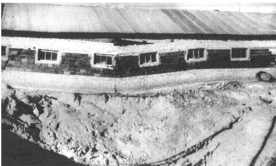
Fig.4.7 Collapse sinkhole on the territory of the Dzerzhinskaya heat and power station (diameter 26 m, depth 5.5 m)
