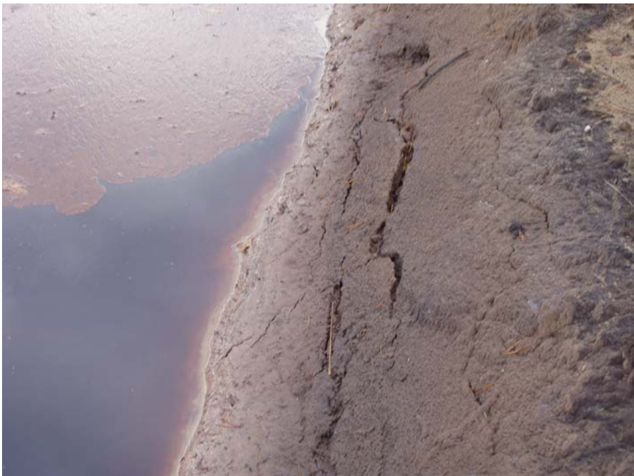
Fig. 1.13 Cracks in the earth slope of the pond bank. There is no insulation layer. The soil is heavily saturated with brown oily liquid
