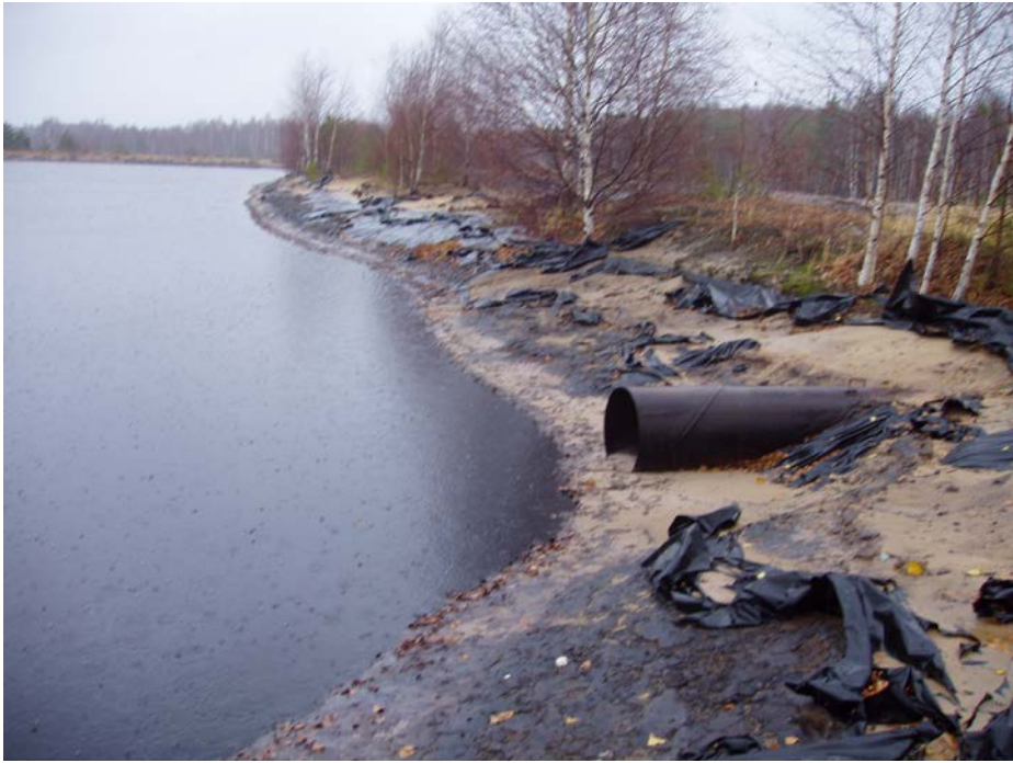
Fig. 1.16 Crossover pipe between ponds with a badly damaged insulation layer
