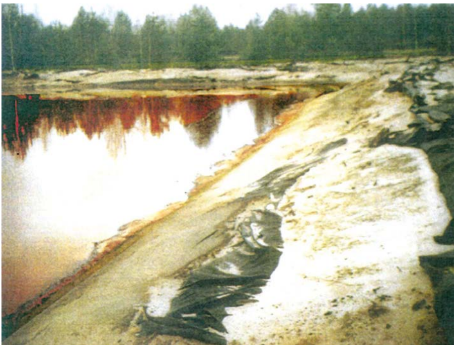
Fig. 1.11 A damaged insulation layer in the form of a black film on the bank of an earth reservoir
